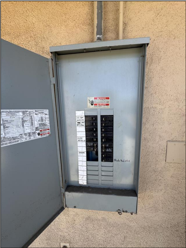
6.3 Item 3 (Picture) Service Panel 3
