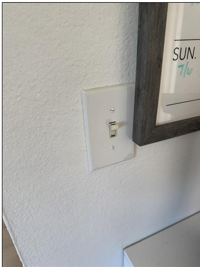
6.6 Item 1 (Picture) Non-Functioning Switch
