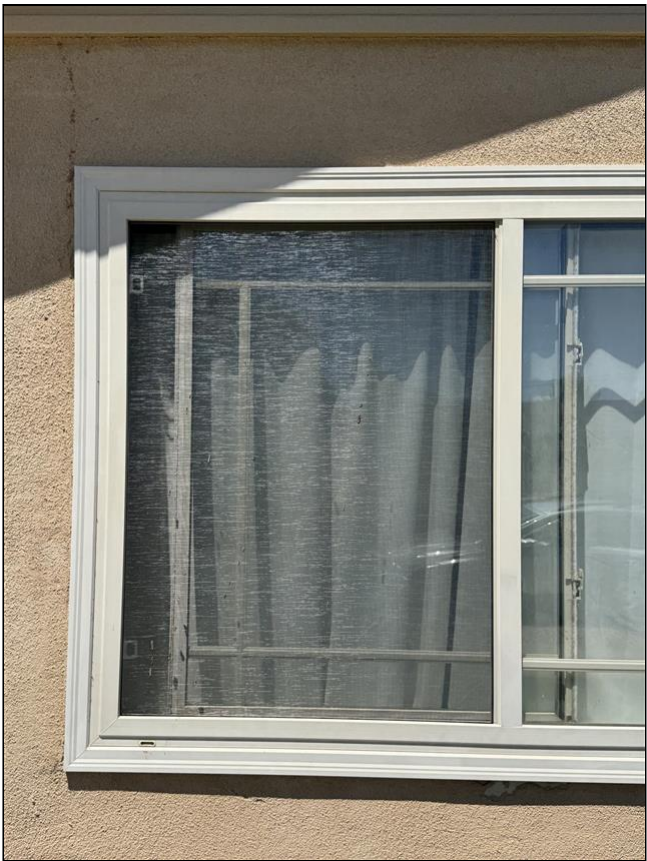
3.1 Item 4 (Picture) Windows 4- Deteriorated Screen
