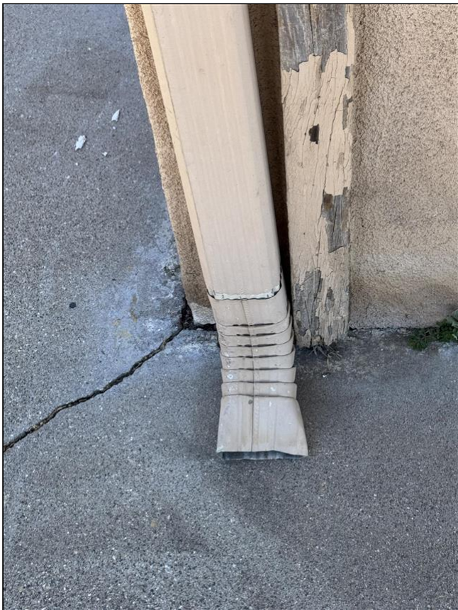
1.2 Item 9 (Picture) Bent Downspout 2
