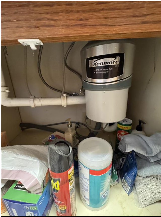
12.6 Item 1 (Picture) Garbage Disposal
