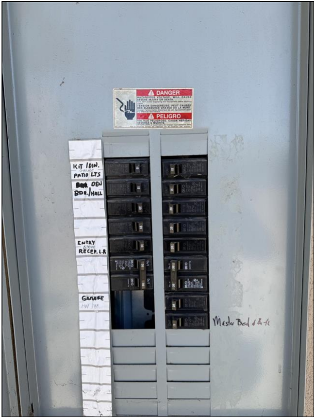
6.3 Item 1 (Picture) Service Panel 1
