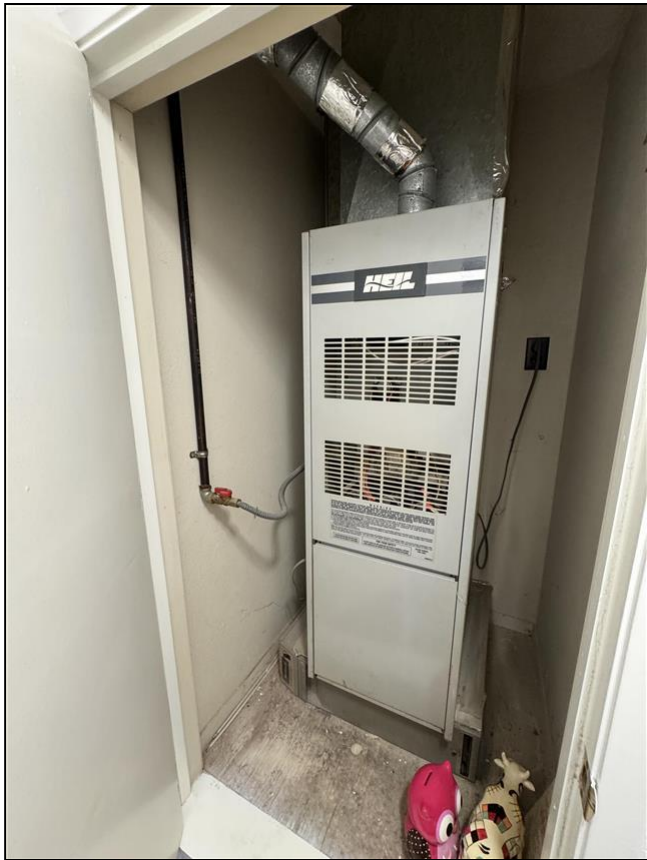
10.1 Item 1 (Picture) Furnace 1
