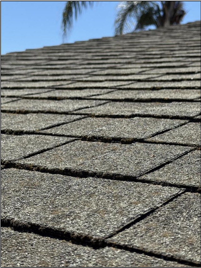
1.4 Item 3 (Picture) Shingles 3
