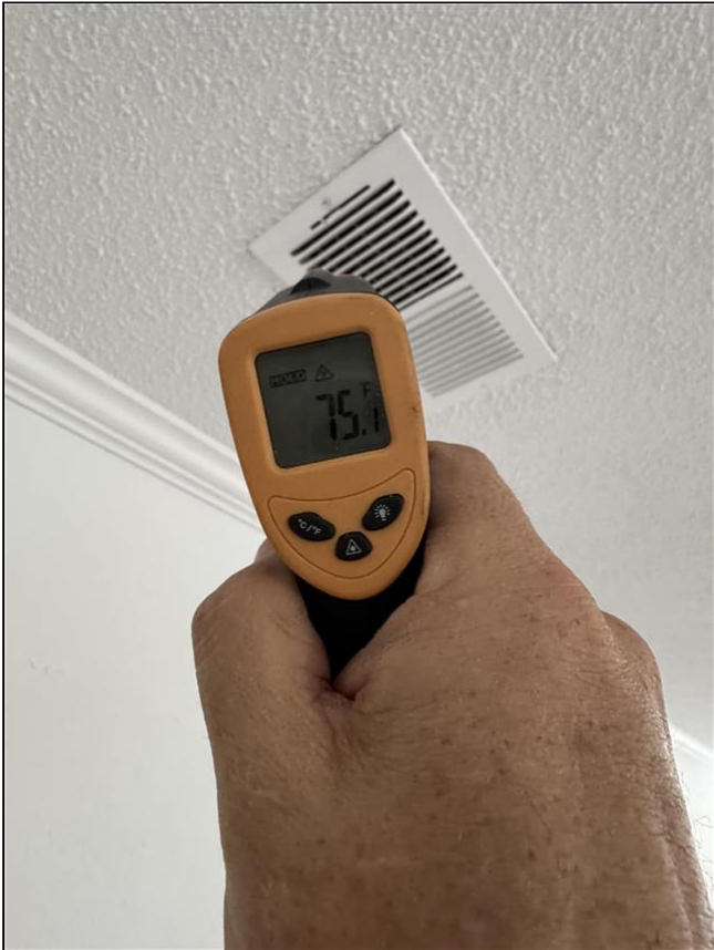
10.0 Item 1 (Picture) Vent Test 1
