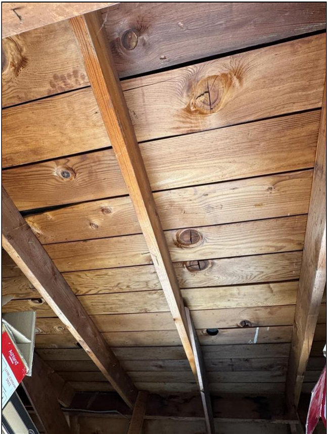
7.3 Item 2 (Picture) Ceilings 1
