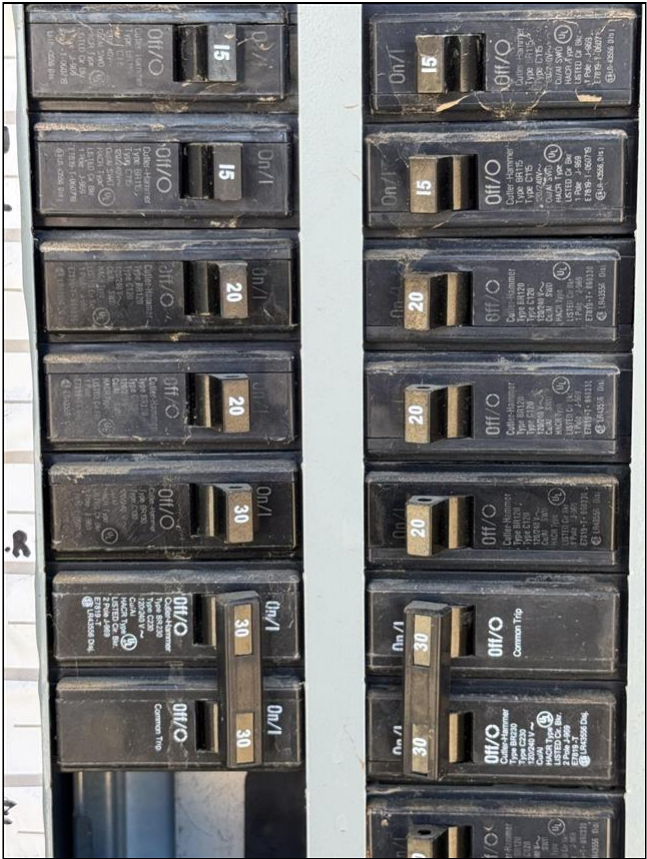
6.3 Item 2 (Picture) Service Panel 2
