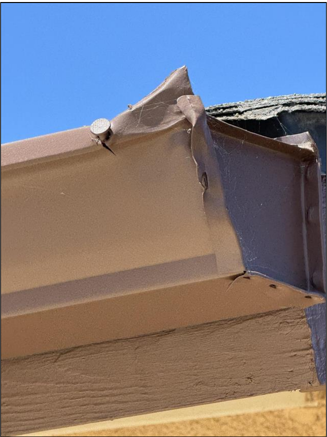
1.2 Item 4 (Picture) Gutter Bent Upward Corner
