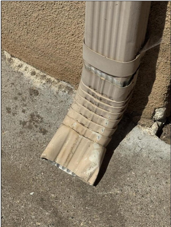
1.2 Item 5 (Picture) Bent Downspout
