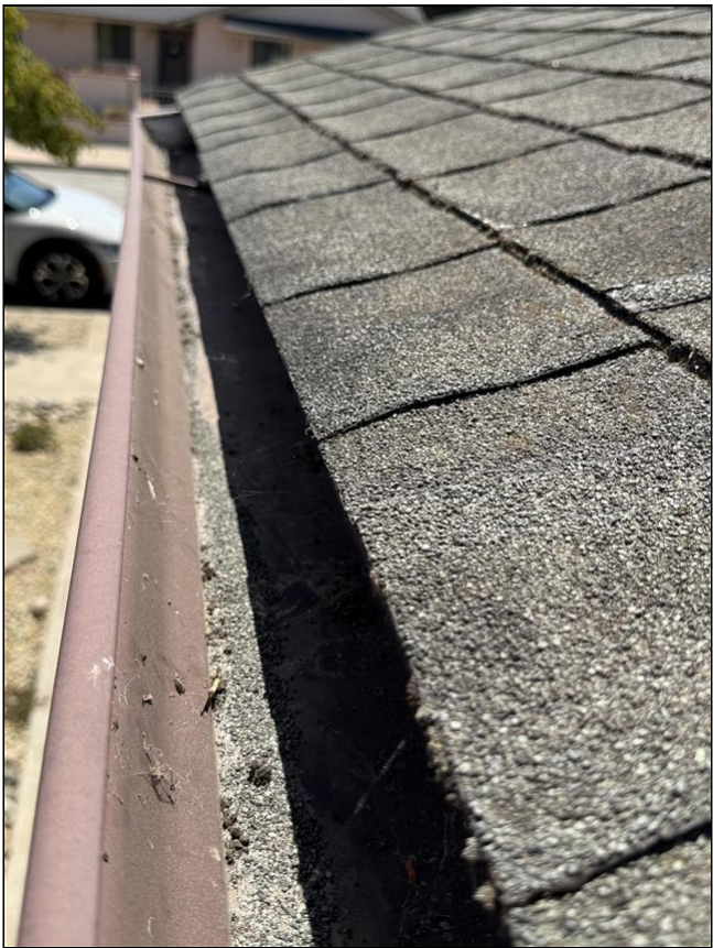
1.2 Item 8 (Picture) Dirty Gutter 3
