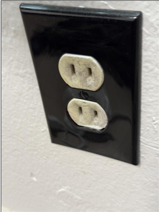
6.4 Item 5 (Picture) Bedroom Loose No Ground
