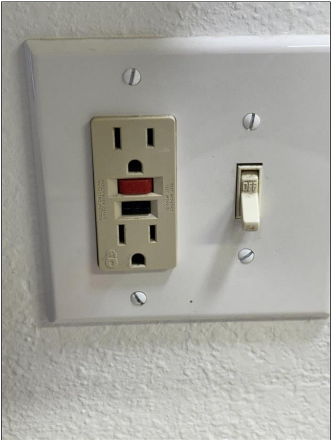
6.5 Item 2 (Picture) GFCI 2
