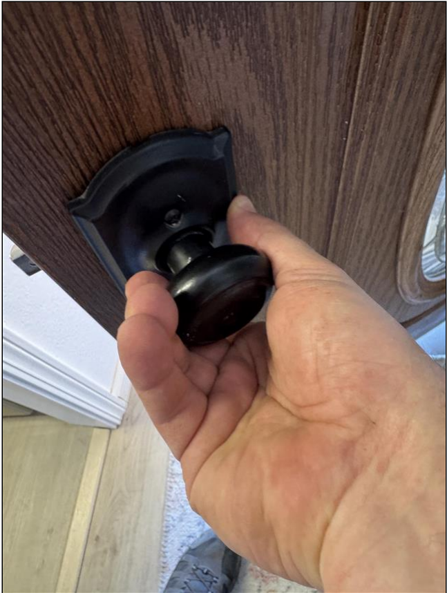
3.0 Item 2 (Picture) Loose Door Handle
