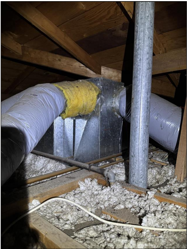
5.1 Item 8 (Picture) Heating System
