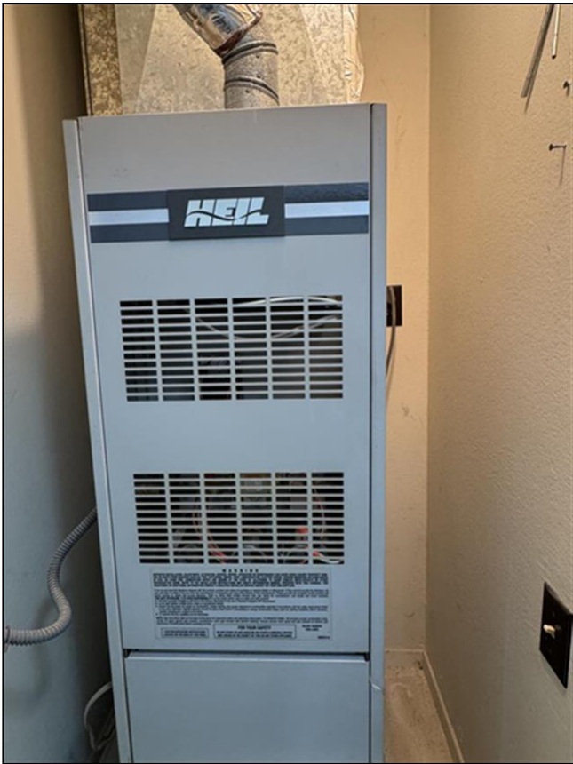
10.1 Item 2 (Picture) Furnace 2
