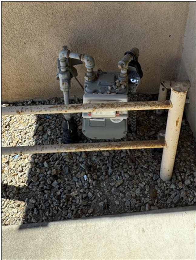
9.4 Item 1 (Picture) Gas Meter and Shut off
