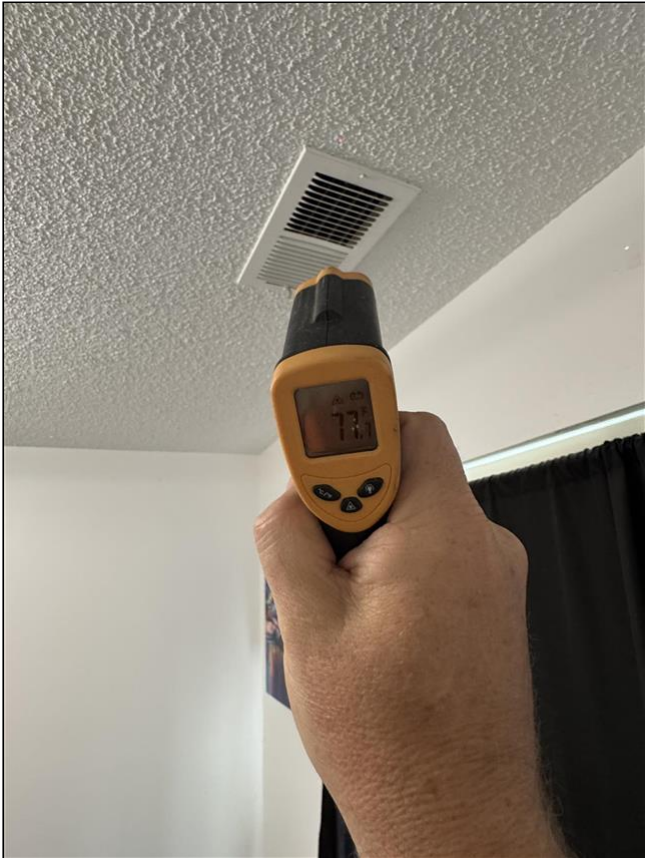
10.0 Item 2 (Picture) Vent Test 2
