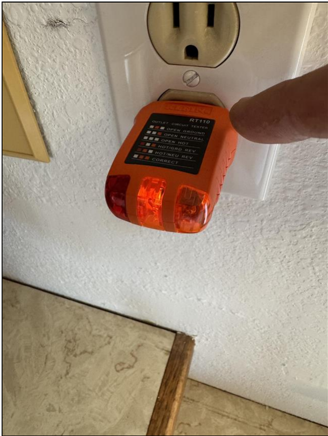
6.4 Item 1 (Picture) Corner Kitchen Receptacle
