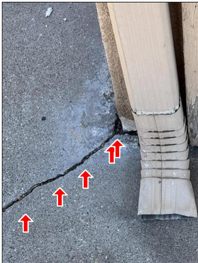
2.2 Item 3 (Picture) Large Crack
