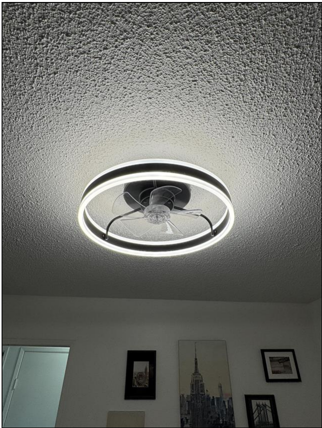
6.7 Item 3 (Picture) Bedroom Light and Fan 1
