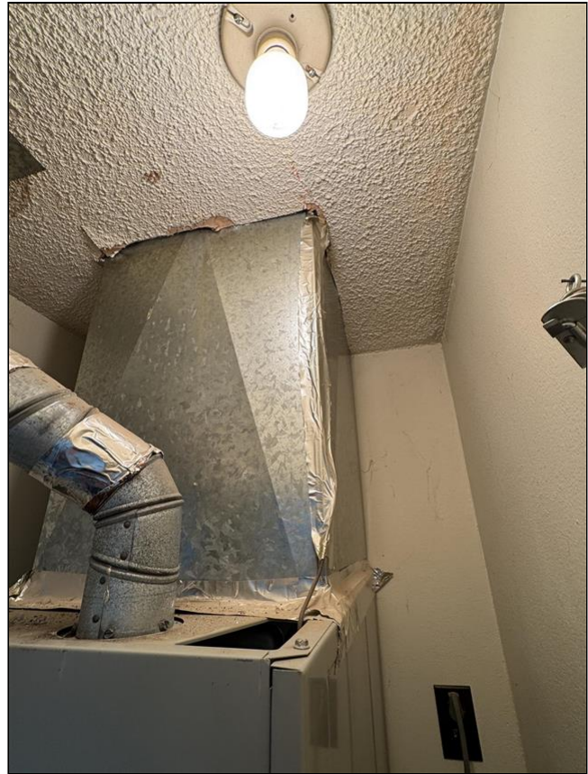
10.1 Item 4 (Picture) Top of Vent Sealed
