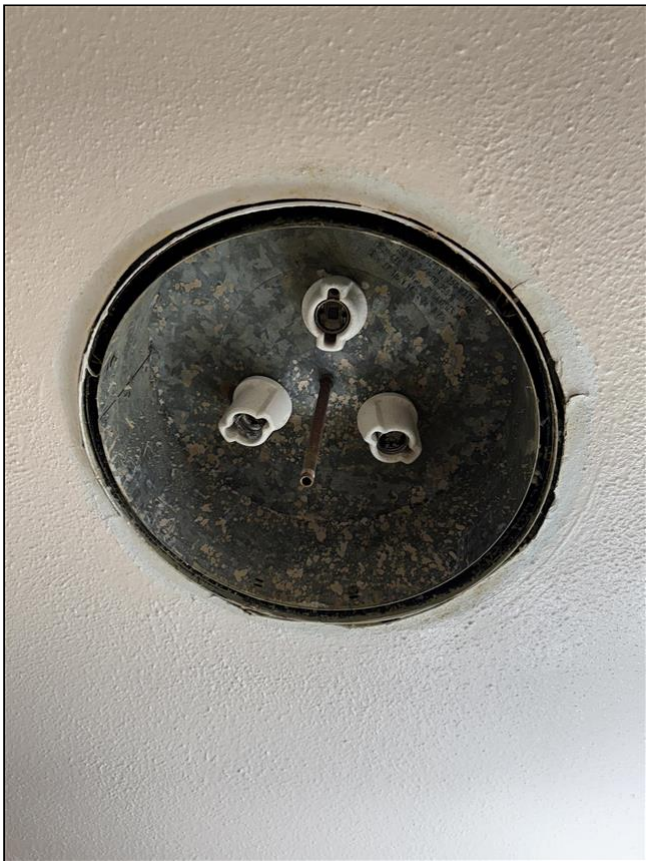
6.7 Item 9 (Picture) Master Bathroom Fixture
