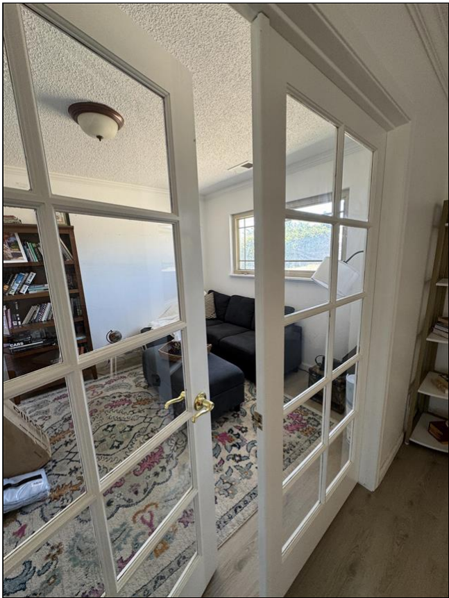
8.4 Item 1 (Picture) Wobbly Doors
