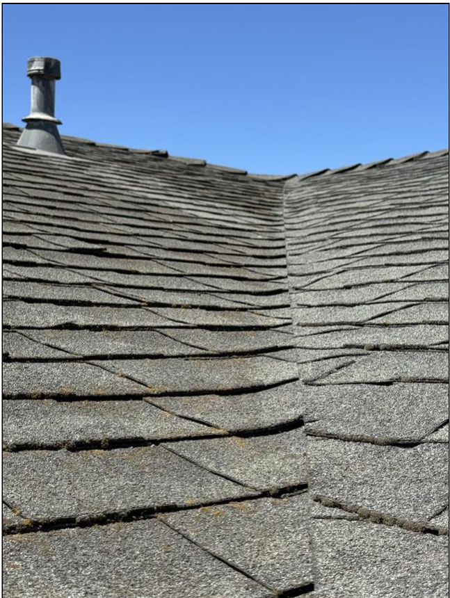
1.4 Item 2 (Picture) Shingles 2
