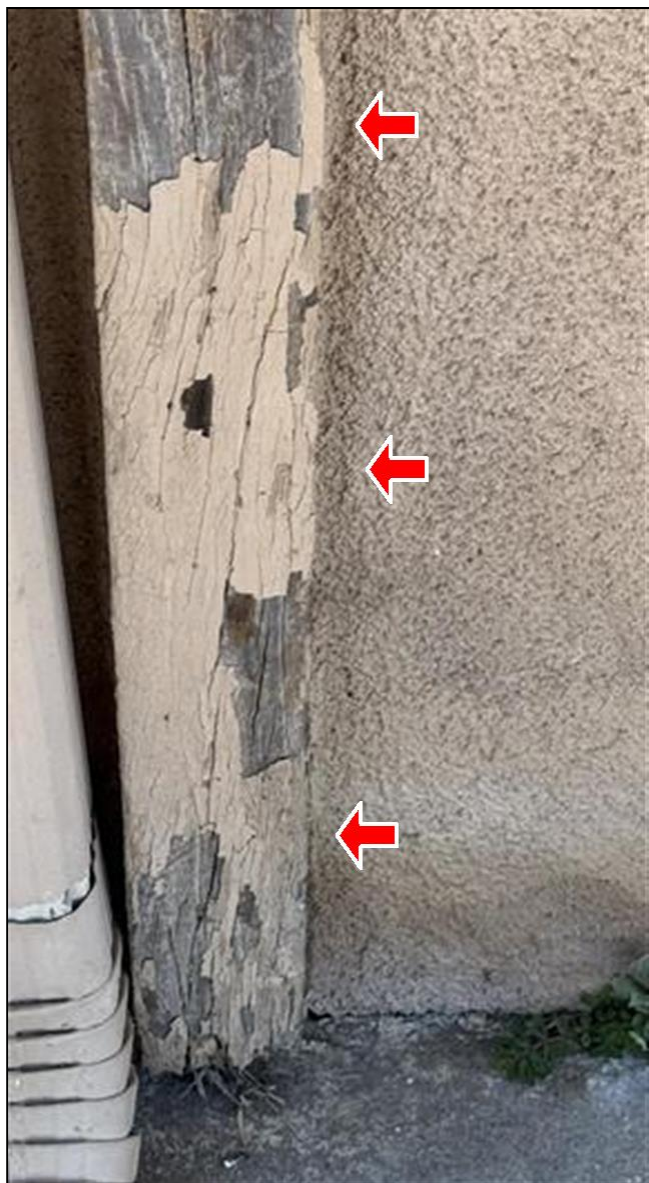
2.3 Item 1 (Picture) Older Wood Trim
