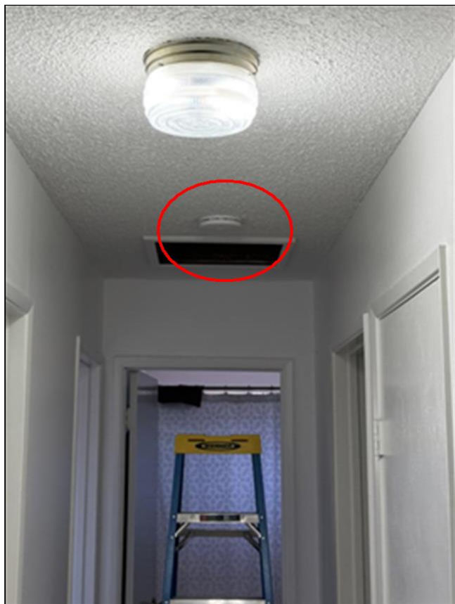
6.8 Item 1 (Picture) Hallway Smoke Detector
