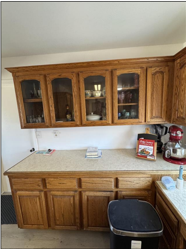
12.4 Item 3 (Picture) Cabinet 3
