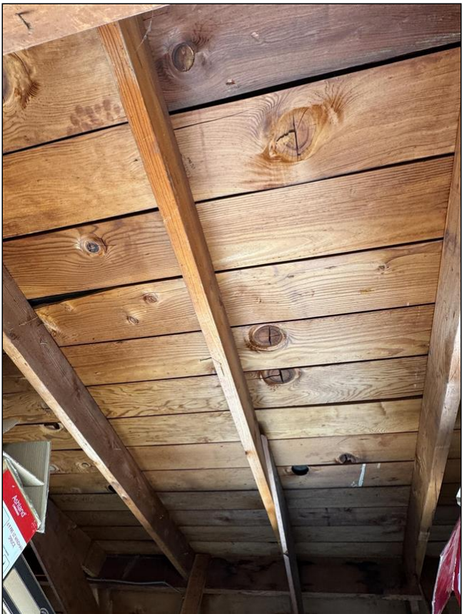
7.3 Item 4 (Picture) Ceilings 3
