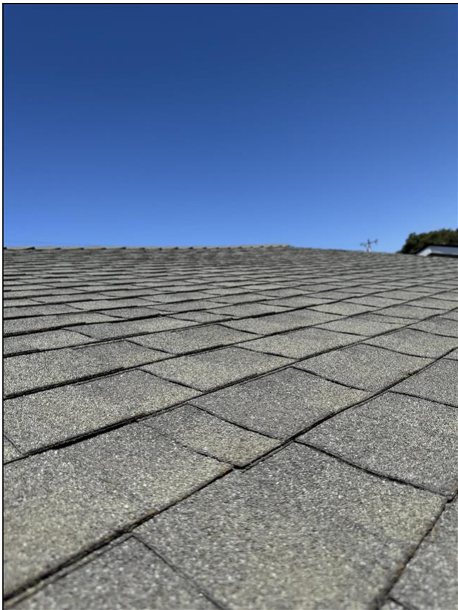
1.4 Item 1 (Picture) Shingles 1
