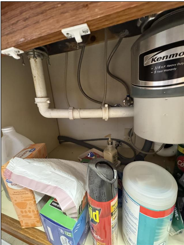
12.4 Item 5 (Picture) Under Sink
