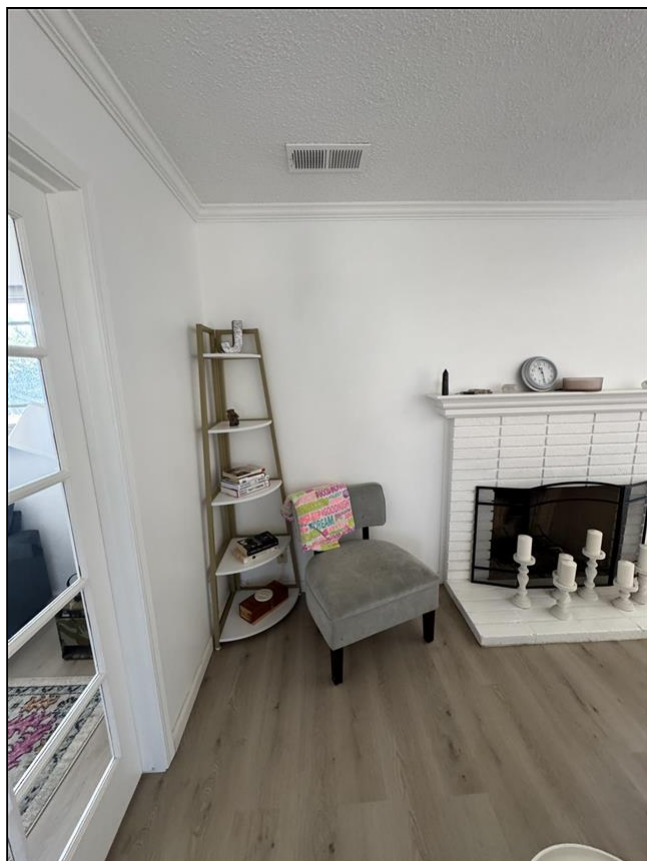
8.2 Item 1 (Picture) Ceilings
