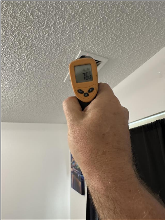
10.0 Item 3 (Picture) Vent Test 3
