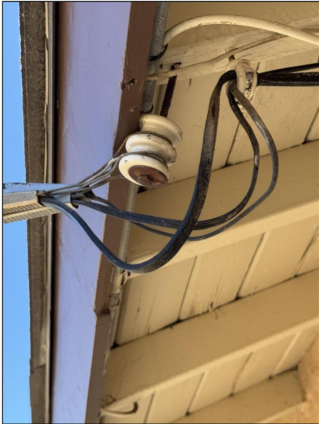
6.11 Item 1 (Picture) Service Drop
