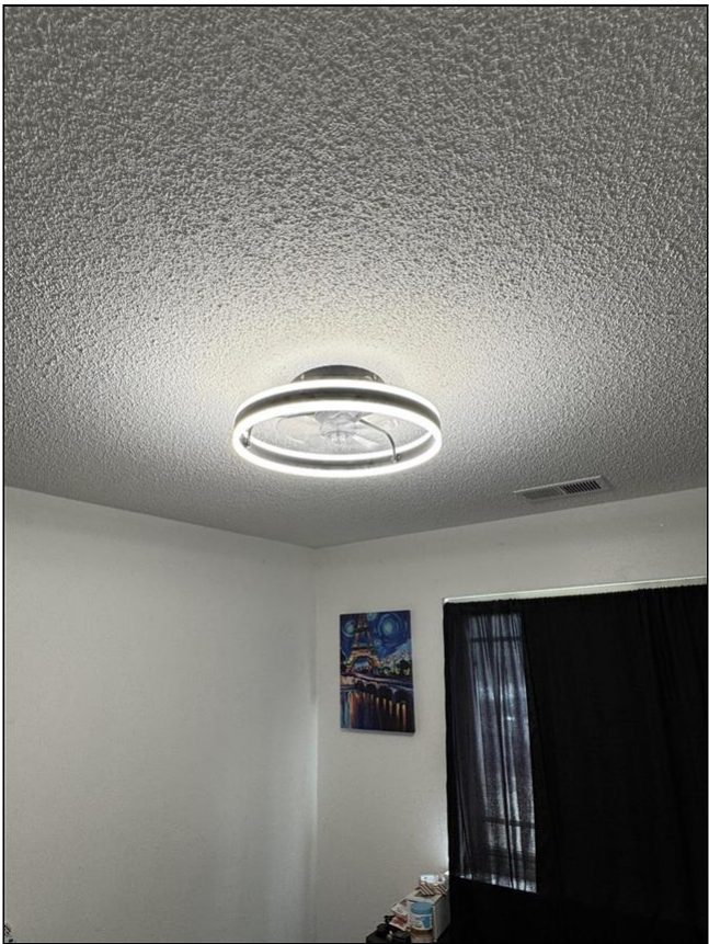
6.7 Item 4 (Picture) Bedroom Light and Fan 2
