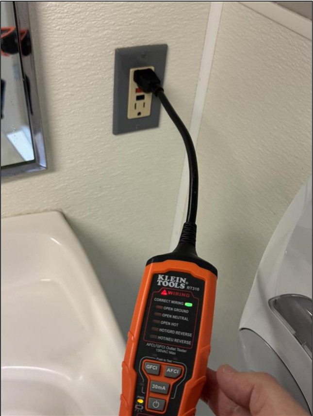
6.0 Item 6 (Picture) Bathroom GFCI Test
