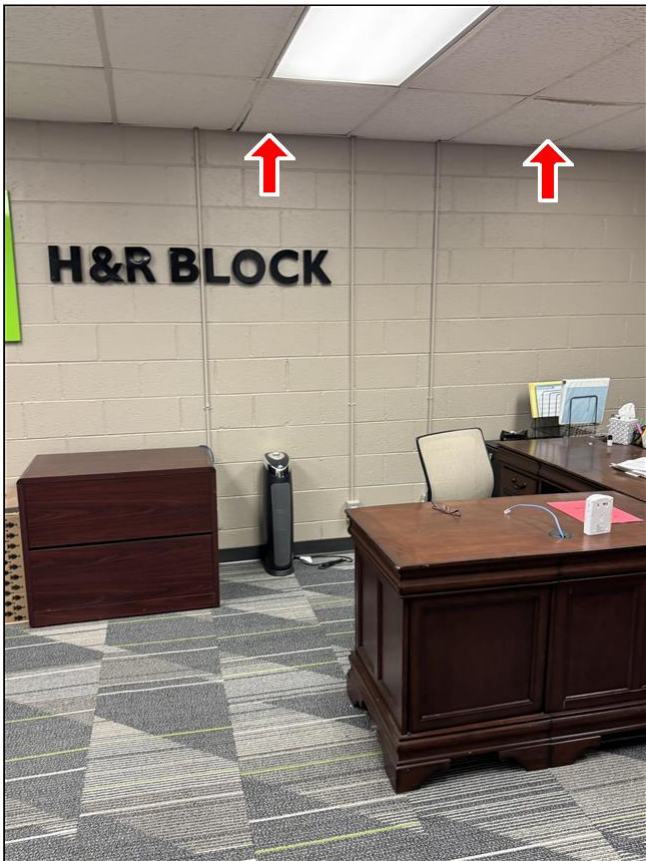
8.1 Item 5 (Picture) Conference Room Ceiling Buckling
