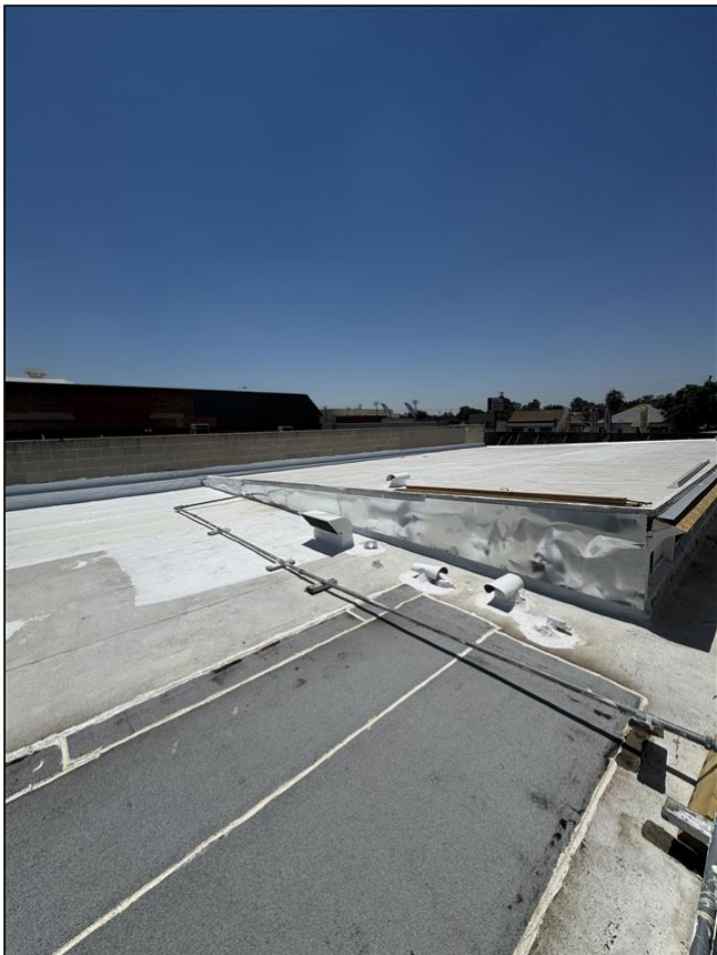
2.0 Item 1 (Picture) Recent Sealing
