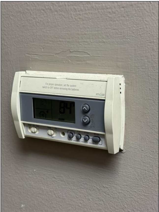
5.0 Item 6 (Picture) Thermostat 2
