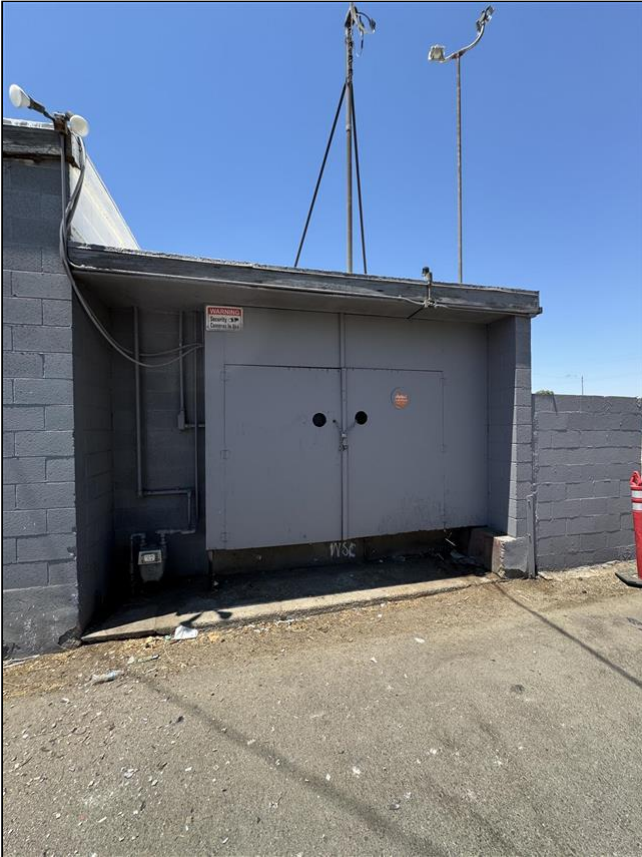
6.0 Item 1 (Picture) Utility Cabinet
