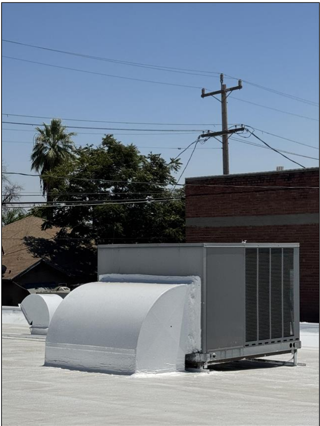
5.0 Item 2 (Picture) HVAC 2
