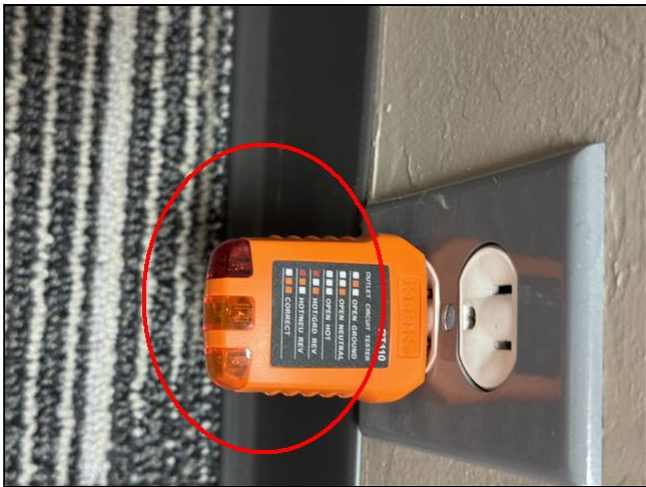
6.0 Item 7 (Picture) End Media Room Test
