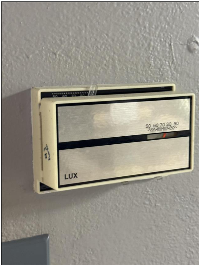
5.0 Item 5 (Picture) Thermostat 1
