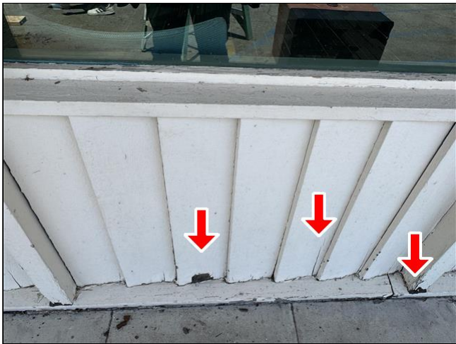
3.2 Item 3 (Picture) Siding Chipping
