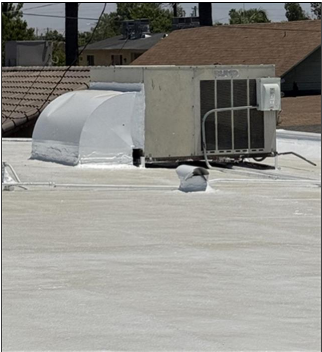
5.0 Item 4 (Picture) HVAC 4
