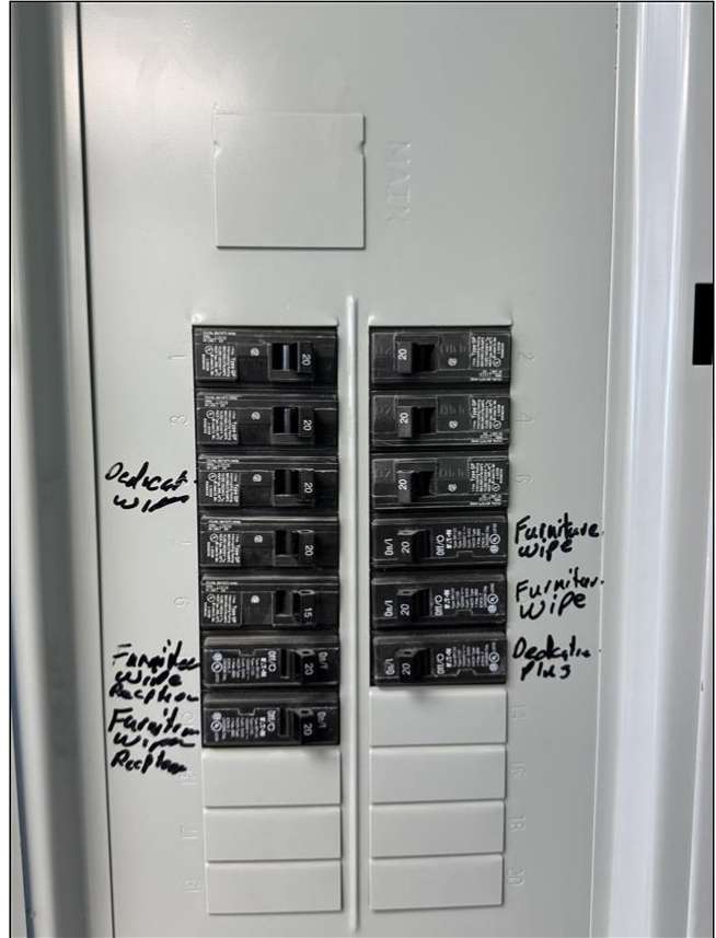
6.0 Item 2 (Picture) Sub Panel 1
