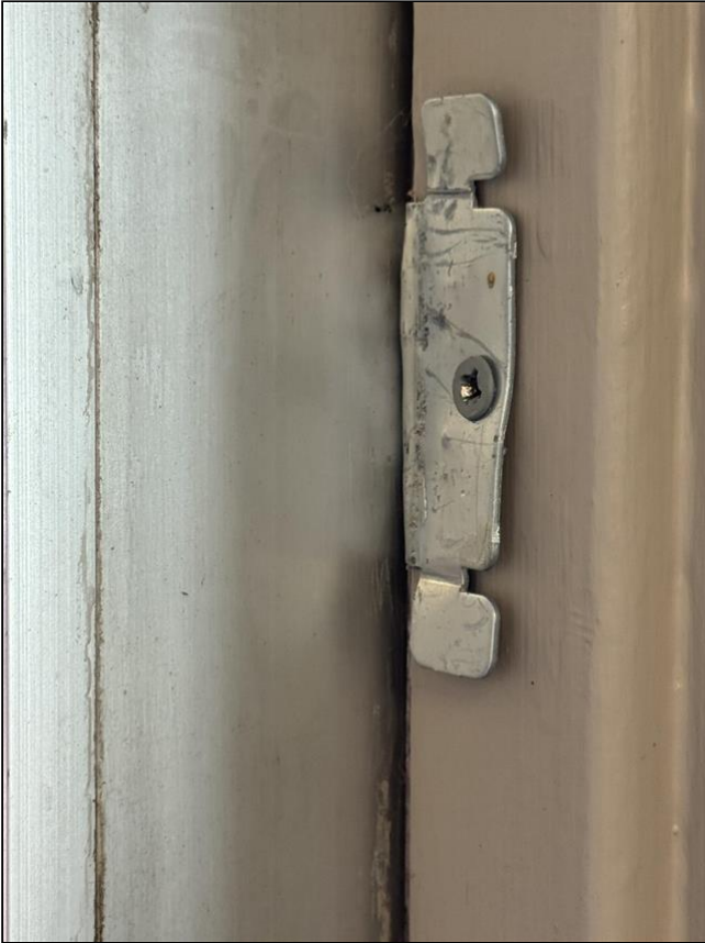
8.4 Item 1 (Picture) Front Door Screwed Shut
