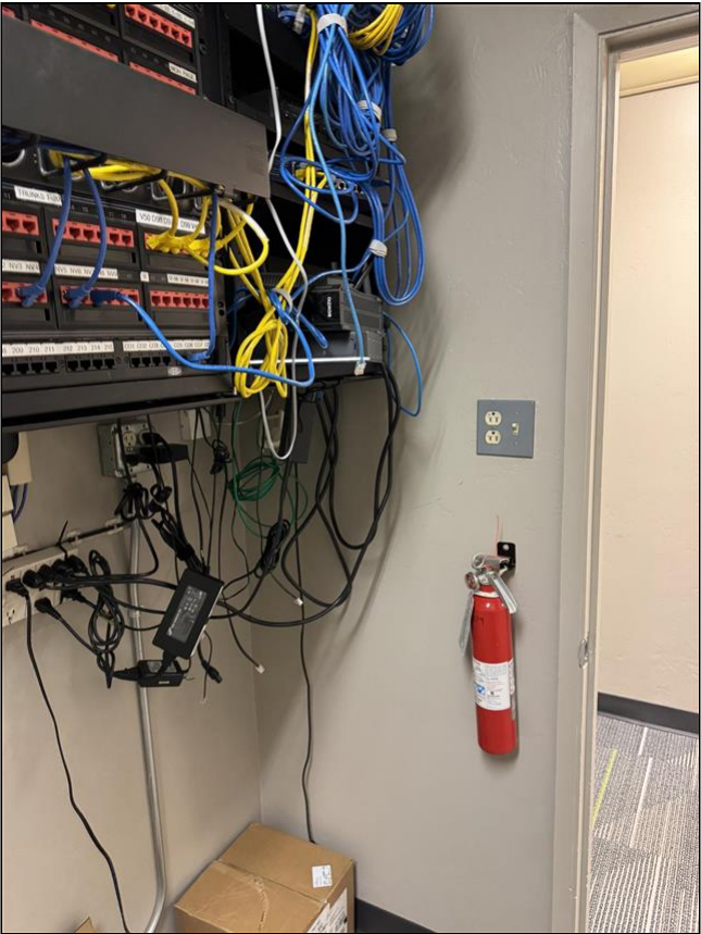
6.0 Item 4 (Picture) Utility Room
