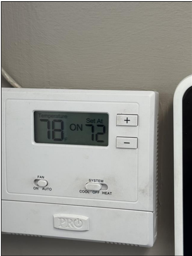
5.0 Item 7 (Picture) Thermostat 3
