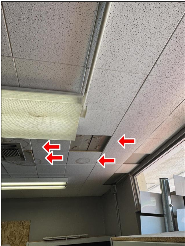
8.1 Item 9 (Picture) Missing Tiles and Leaks Storage
