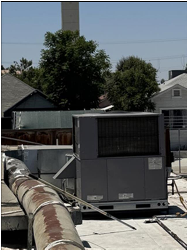
5.0 Item 3 (Picture) HVAC 3
