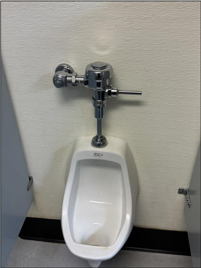
7.0 Item 7 (Picture) Urinal
