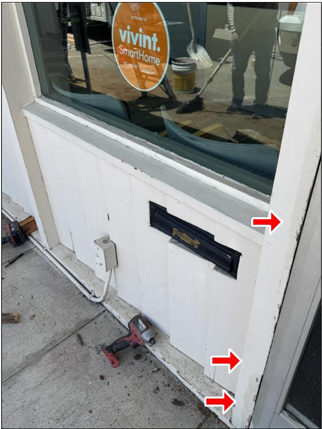
3.2 Item 4 (Picture) Siding Chipping 2
