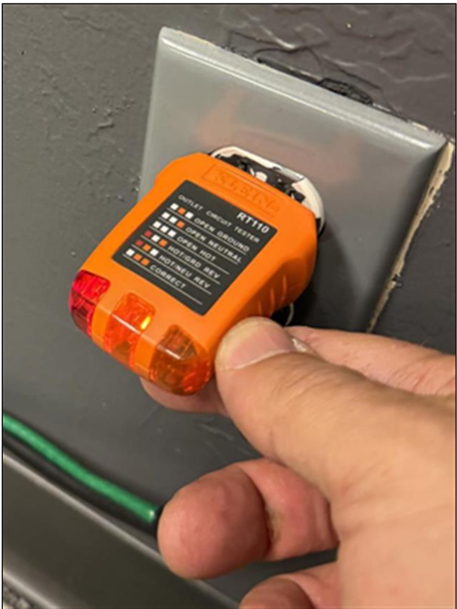
6.0 Item 10 (Picture) Media Loose Bad Ground 2
