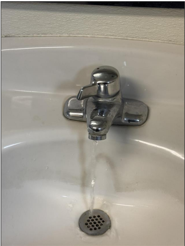
7.0 Item 6 (Picture) Sink 3
