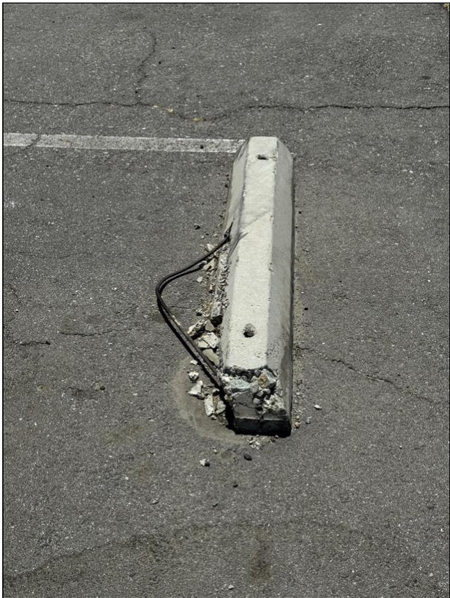
4.0 Item 1 (Picture) Broken Parking Block
