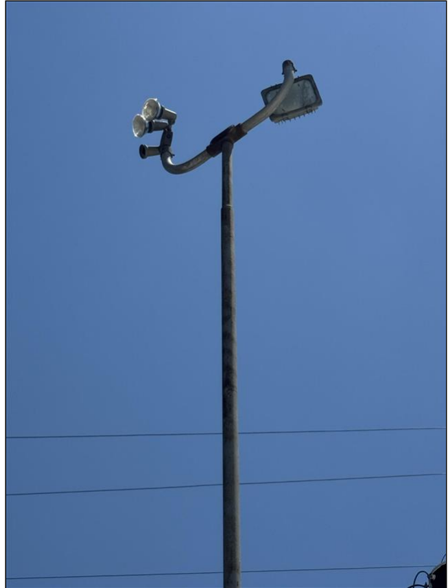
3.6 Item 2 (Picture) Non Working Lights
