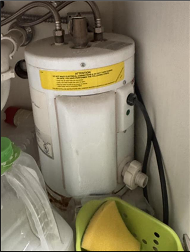
7.0 Item 9 (Picture) Electrical Water Heater
