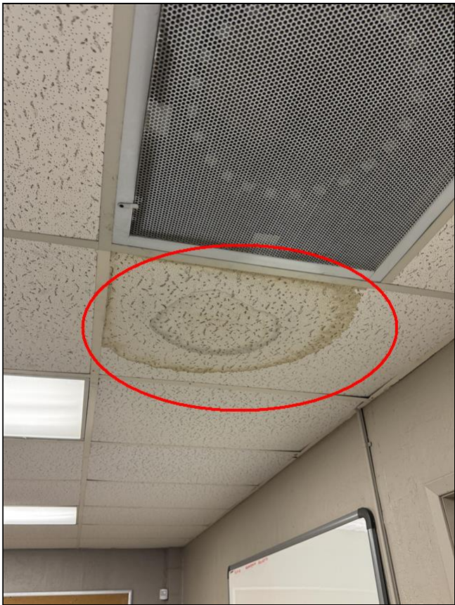
8.1 Item 7 (Picture) Larger Leak CR
