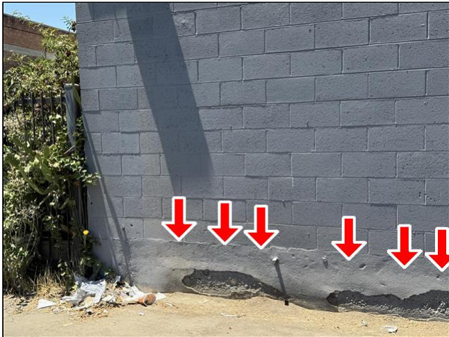
3.2 Item 1 (Picture) Damaged Masonry
