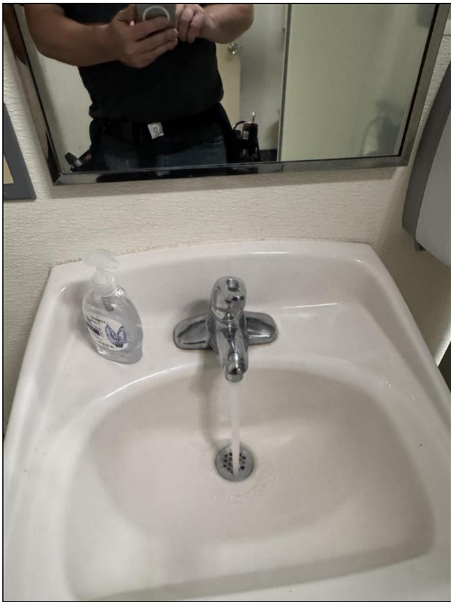
7.0 Item 3 (Picture) Sink
