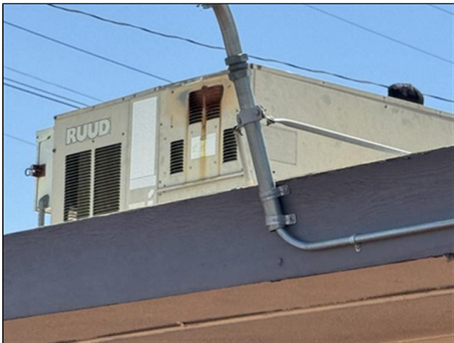
5.0 Item 1 (Picture) HVAC 1
