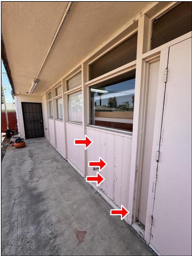
3.2 Item 5 (Picture) Siding Chipping 3
