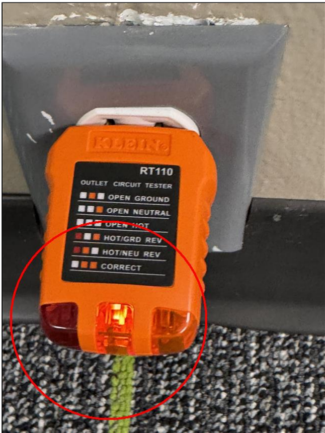
6.0 Item 9 (Picture) Media Loose Bad Ground
