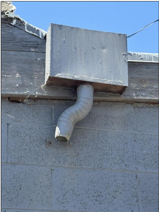
2.2 Item 5 (Picture) Incomplete Drainage
