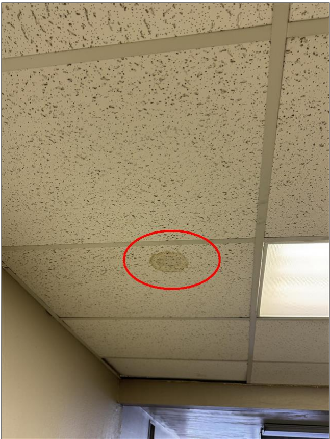
8.1 Item 6 (Picture) Small Leak CR
